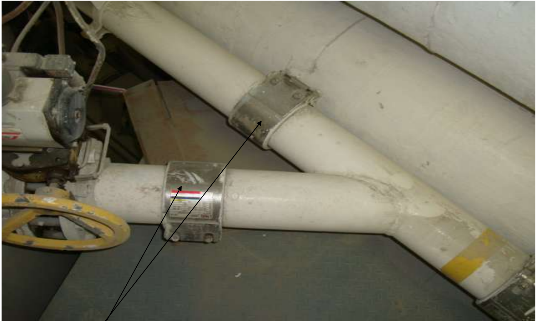
The same clamp coupling arrangement in place at another location on the bulk discharge system
