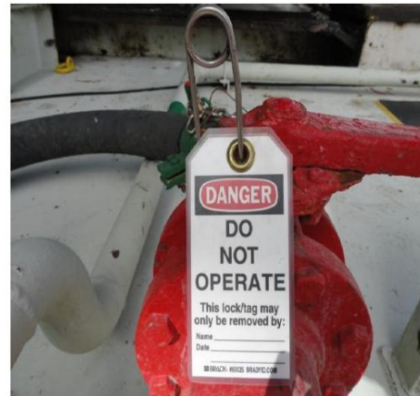
Pic 1: shows unsafe practice by using safety pin to effect mechanical lock out on a valve and the tag was not filled out as required.
